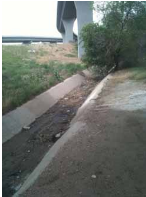
Photo 11 — The concrete lined ditch north and east of US 6 and I-25. No wetland plants or hydric soils are present; it is just filled with trash and mud.
